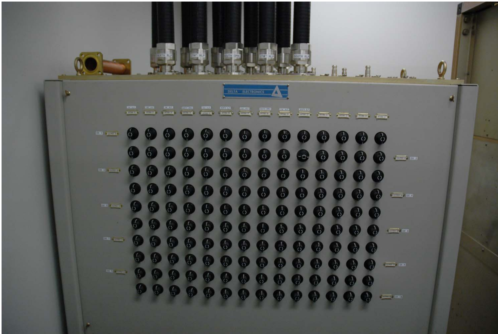
The Antenna Switch Matrix
